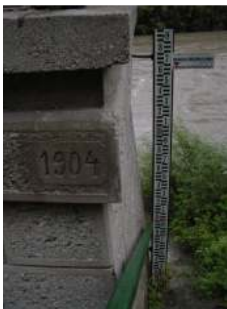
Slika 2. Oznaka leta postavitve temelja hidrološke postaje in najvišje izmerjene gladine vode (foto: Arhiv ARSO) Figure 2. Sign of year of building the gauging station and mark of the highest water level (Photo: Archives of ARSO)
